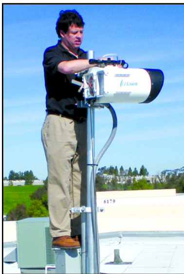
▲ A Loea employee installs the Loea L1000 system at a site in California.
